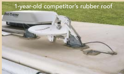
1-year-old Winnebago fiberglass roof
